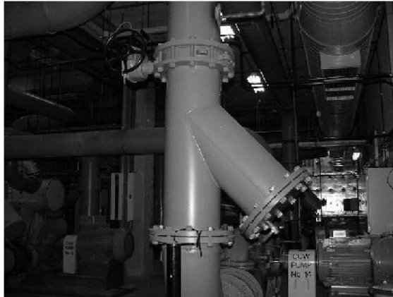
Figure 8.8 A Y-type suction strain in the pump suction
